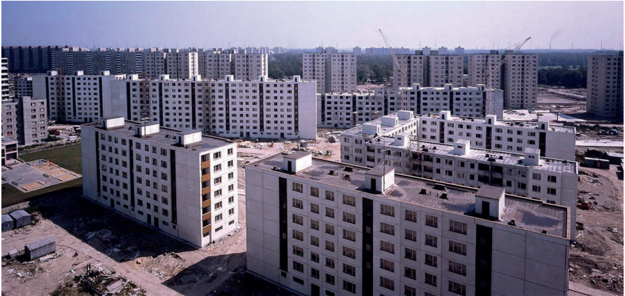
Fig. 4 – Residential district under construction in Bratislava (Slovakia) in the 1970s. The common urban planning, technological and material choices have made the residential districts of the European suburbs very similar to each other, with fairly comparable architectural, material and performance degradation phenomena. Due to the lack of immigration from non-European countries since the 1970s, today in the main cities of Eastern Europe the inhabitants are originally from the place and are generally the owners of the apartment in which they live.
