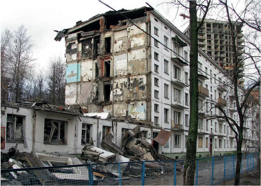
Fig. 1 – Demolition. Moscow district in 2012: in the former Soviet Union and other countries the main strategy is destroy the old prefabricated buildings to leave free space for new residential neighborhood.
